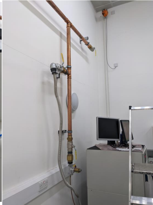
BMPC outlet also attached, with T-ed off NRV. Stainless steel bellows attached to magnet outlet during fill.
