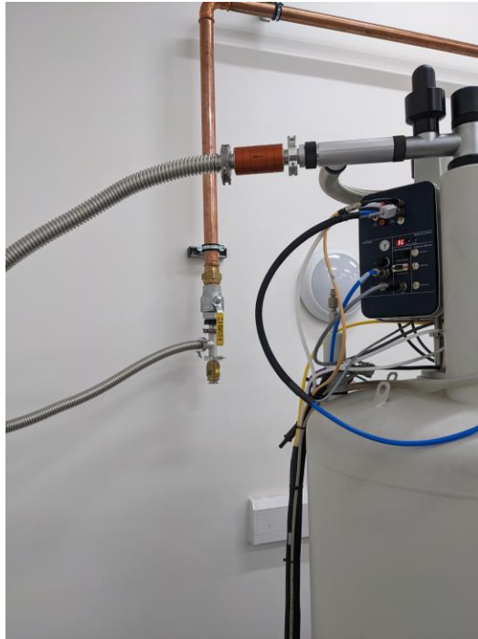
Magnet connections through NRV to stainless steel bellows. Over-pressure managed by 20mbar NRV T-ed off at wall
